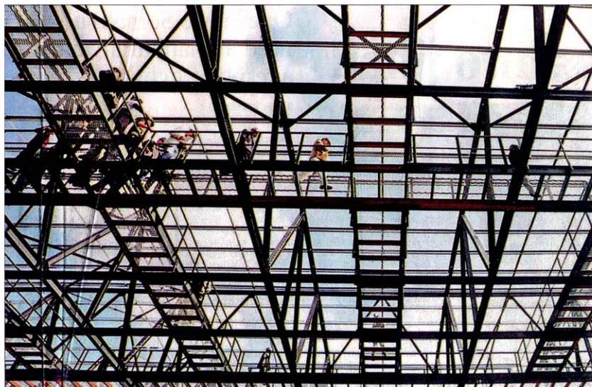
HOLDING UP: Trade and Industry Minister Rob Davies and Cape Town Film Studios head Anant Singh inspect the studio under construction near Faure. It will be ready by July to produce its first movie.
